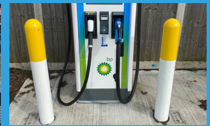
A barrier around a public rapid chargepoint
