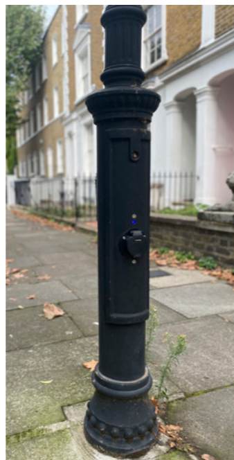
◀ A lamppost charger on a residential street.
