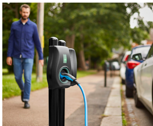
◀ A chargepoint on a residential street.
