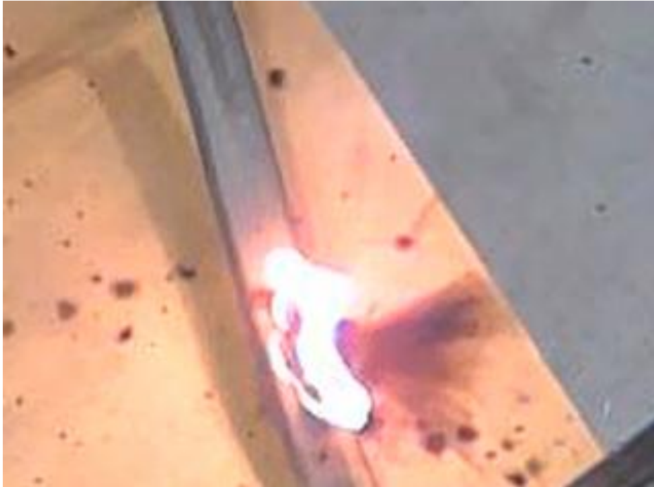
Figure 1-2: ABDX007 (RCBO) PVC Insulation Cable Insulation Flames Following Prolonged Arc
