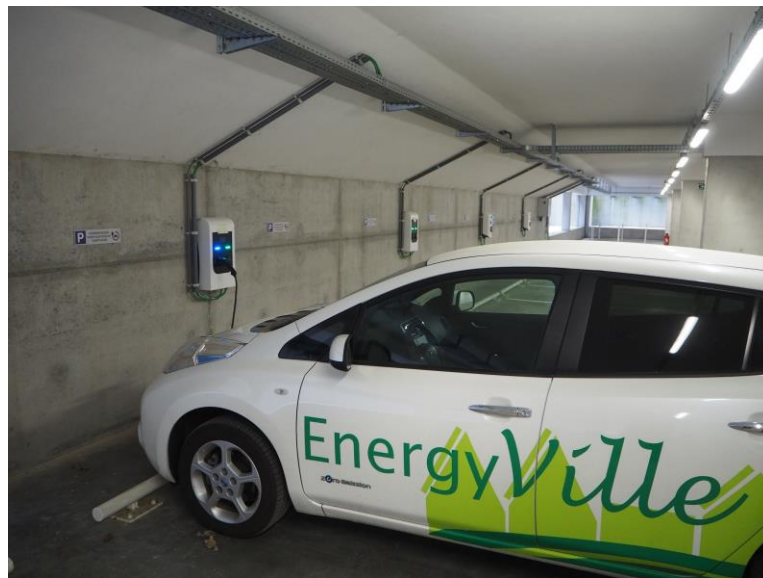
Figure 46 -EnergyVille office building: EV charging equipment
