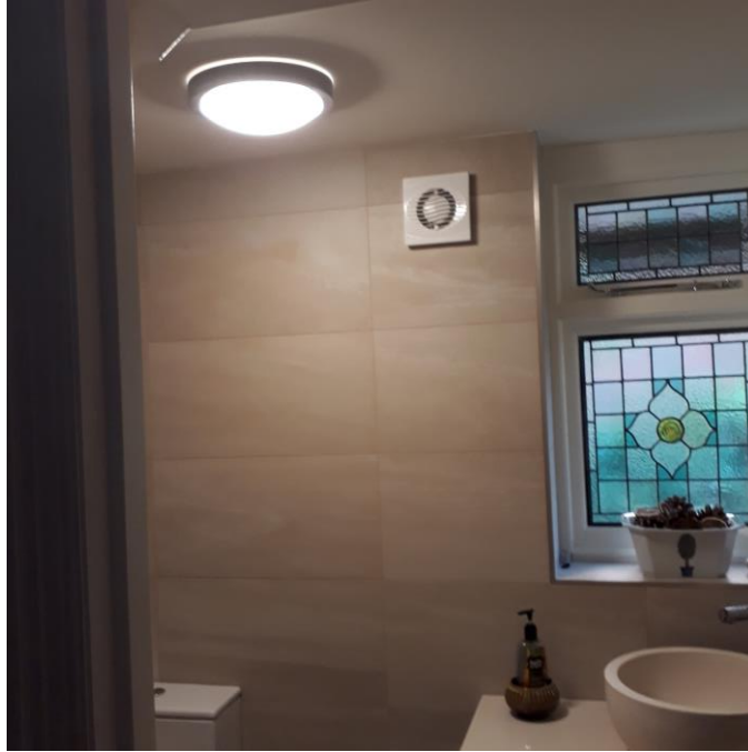
Figure 39 -Presence detection lighting via a motion sensor
